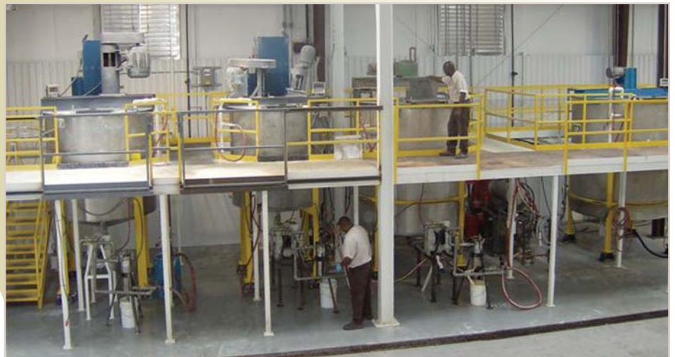
New Liquids Processing Plant
